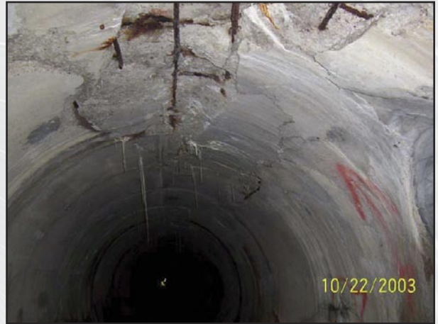
CRACKED AND CORRODED RIGID SEWER PIPE
